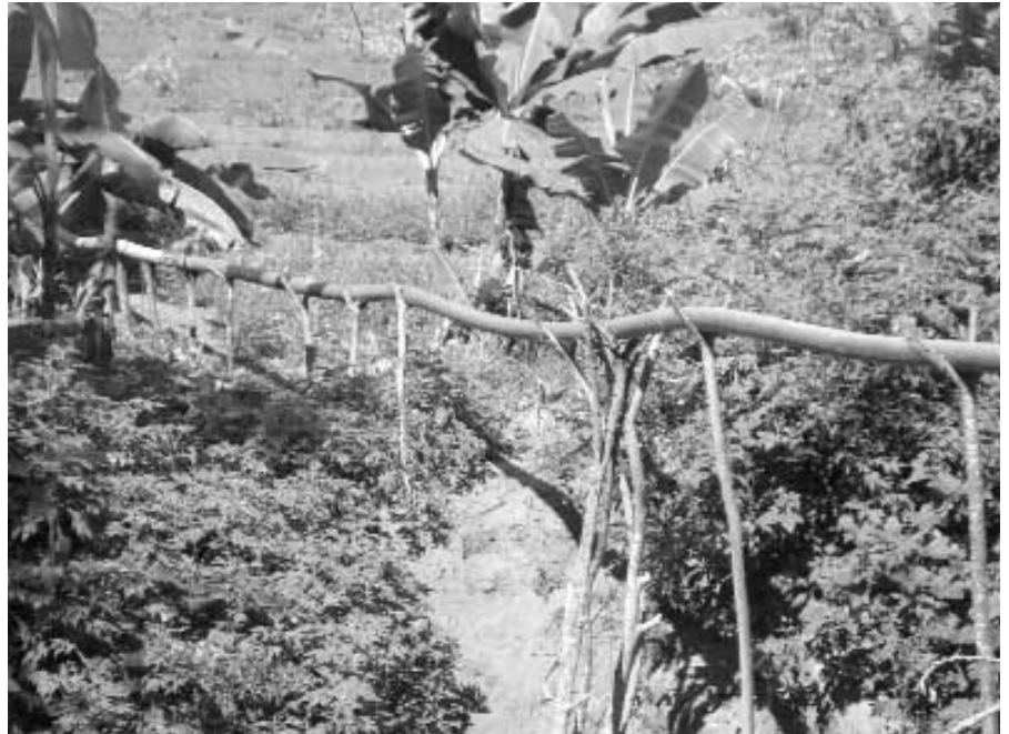
Irrigation piping for the ginger terraces
